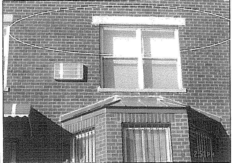
Picture 4 – Bulge in brick veneer extends the length of building exterior parallel to window lintel.
