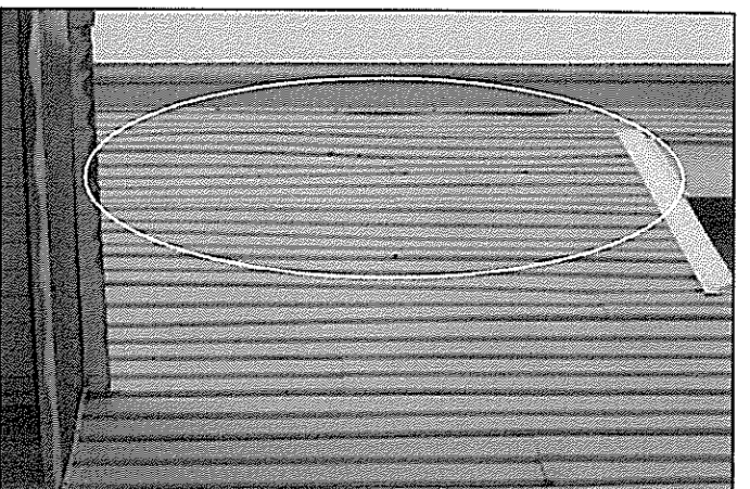
Picture 12 – Rear exterior siding improperly installed. Extensive bulging observed throughout exterior. No separation of siding between attached building.
