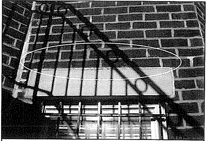
Picture 8 – No weep holes observed for proper drainage.
