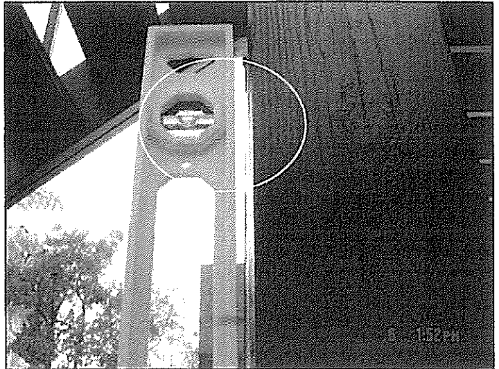
Picture 12 – Facing west. Picture shows large gap between level at plumb and out of plumb column.
