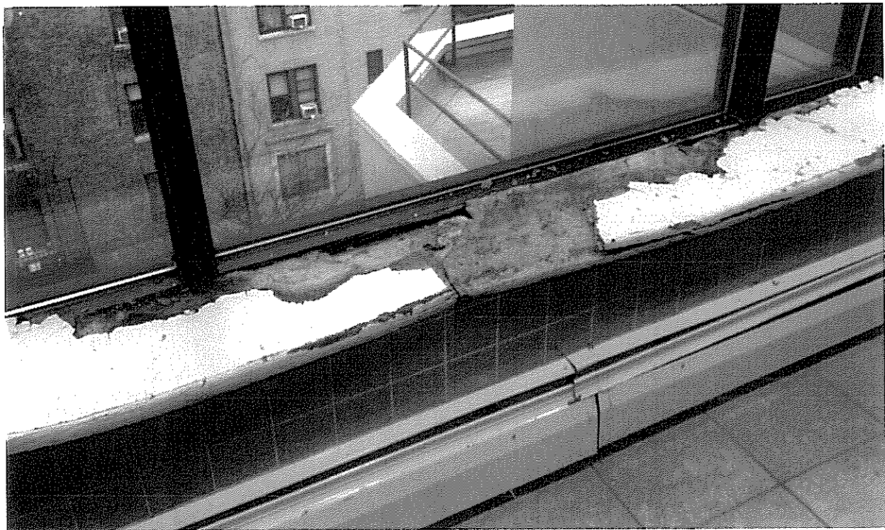
Water damage from untreated leak in hallway
