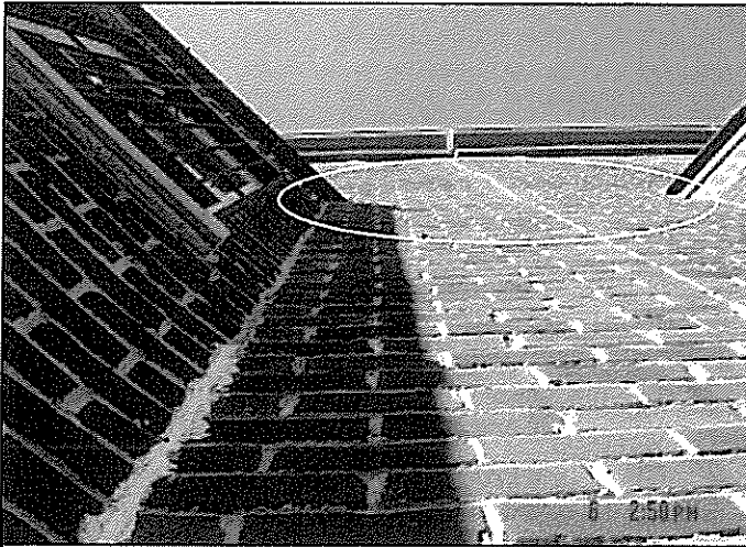
Picture 1 – Large bulge in brick veneer above second story bump out.
