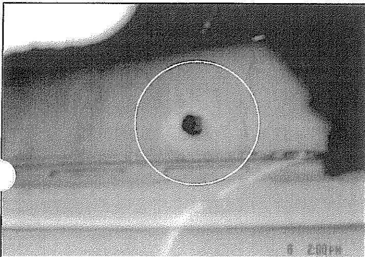
Picture 15-- Facing north. Exterior vinyl siding removed to showing non exterior grade siding. Inspection hole reveals no insulation.
