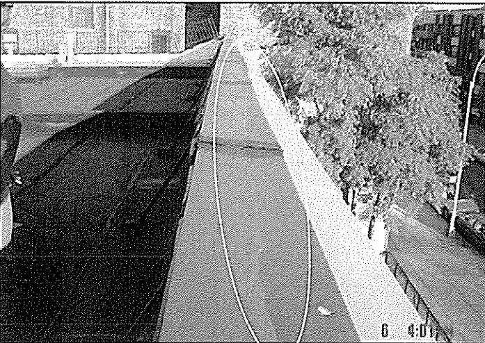
Picture 21- Facing east – damage along entire parapet cap.
