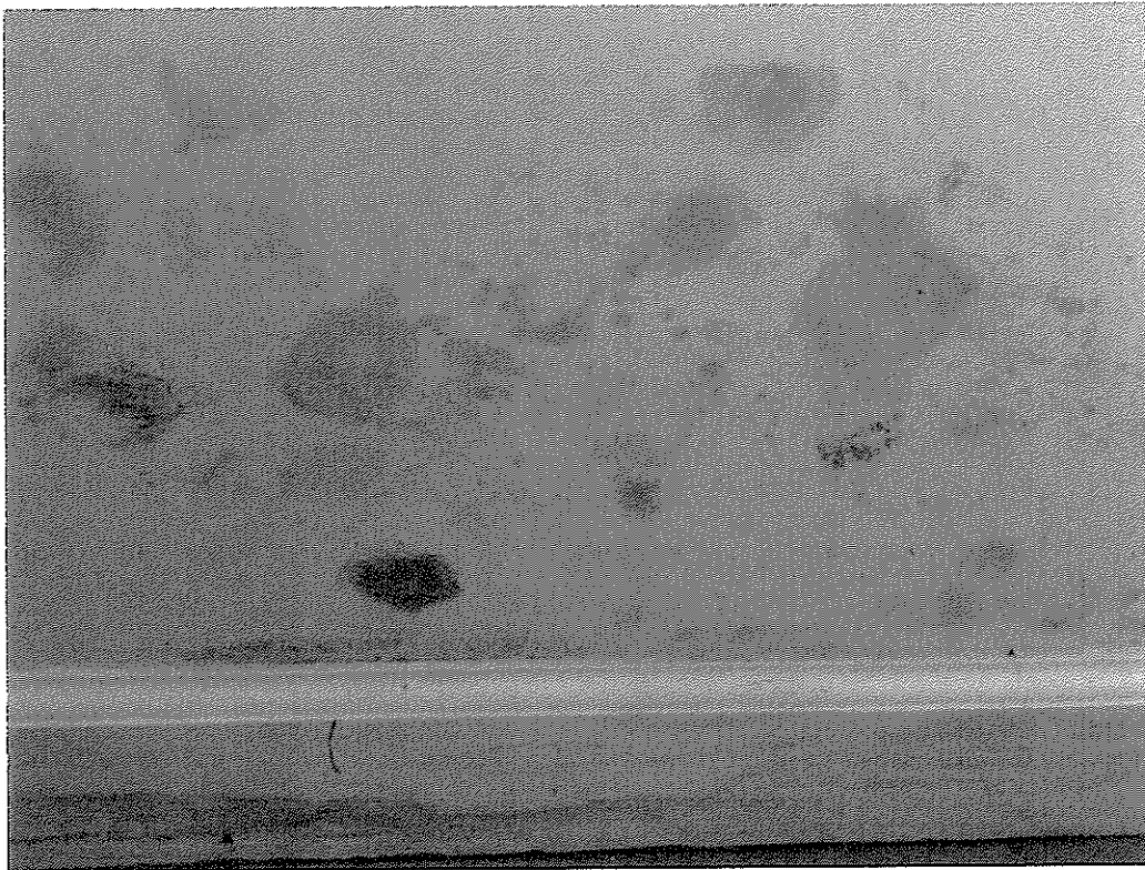
Mold on the bedroom of a HPD homeowner.
