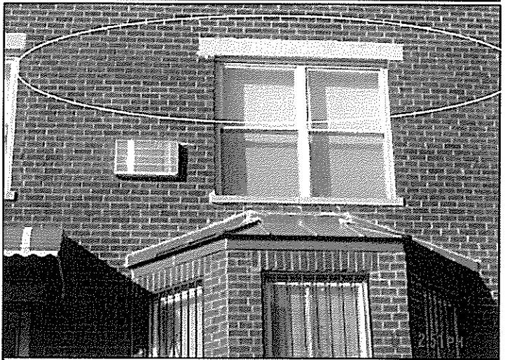
Picture 4 – Bulge in brick veneer extends the length of building exterior parallel to window lintel.
