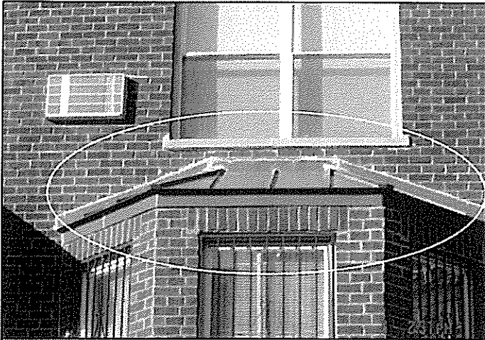
Picture 3 – Liberal use of caulking along cap for bump out. This area corresponds to interior damage and repairs.
