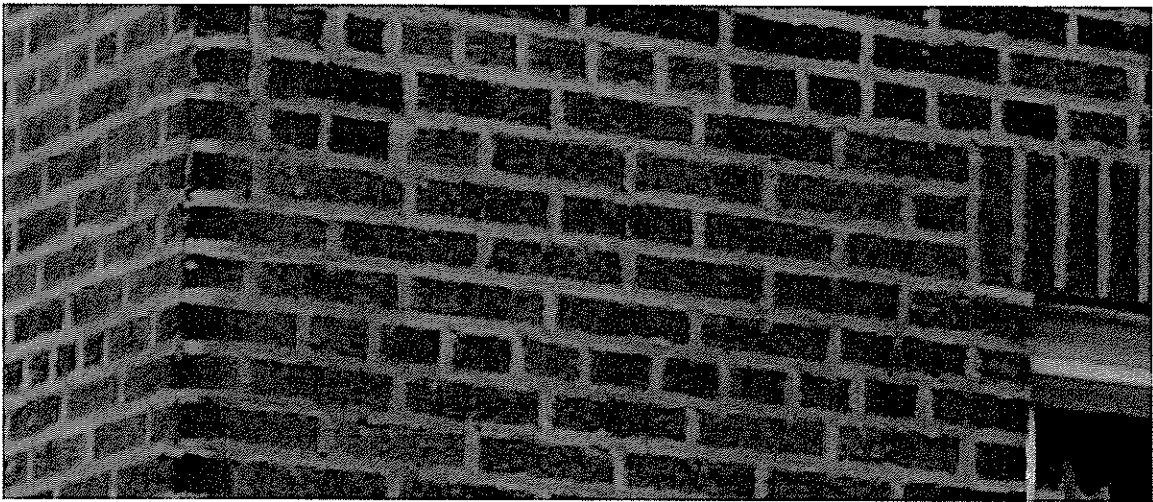
2.3.1 All brickwork of the main structure repointed flush, not the original struck and/or raked joints, and the mortar texture and color are not the original.
