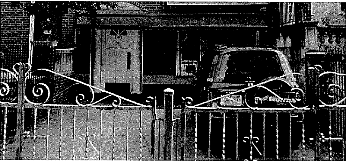
2.2.1.1 Automobile parking relocated from the original interior garage to the front yard, and contrary to the original design poses environmental, fire, health and safety hazards to the property and adjoining properties.
