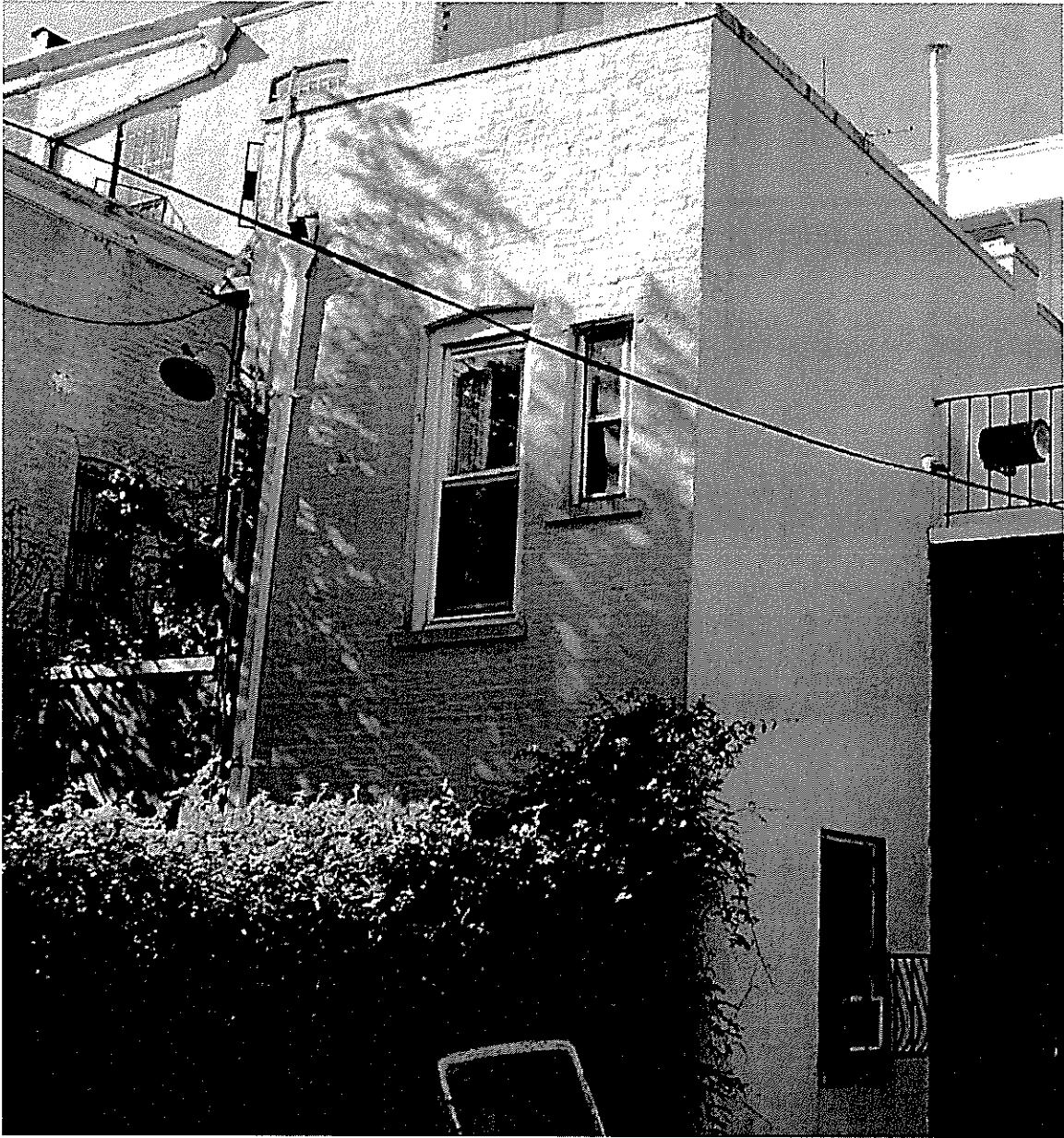
2.2.2 East (rear) Alterations. Lot line window at first floor north is not original and poses hazard to the adjoining property. Air-conditioner and security grille encroach on adjoining property. None of the original paint on painted elements remains and window sash and frames are pre-finished metal.
