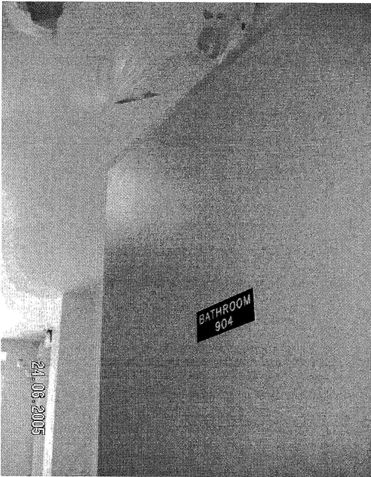
Fig.____. Flooding in common use bathroom 904 from superintendent John Lopez' apartment located on the 10th floor. Management and Adult Protective Services accused a female tenant of causing the "flooding". Capitol Hall S.R.O. Dated: June 24, 2005.
