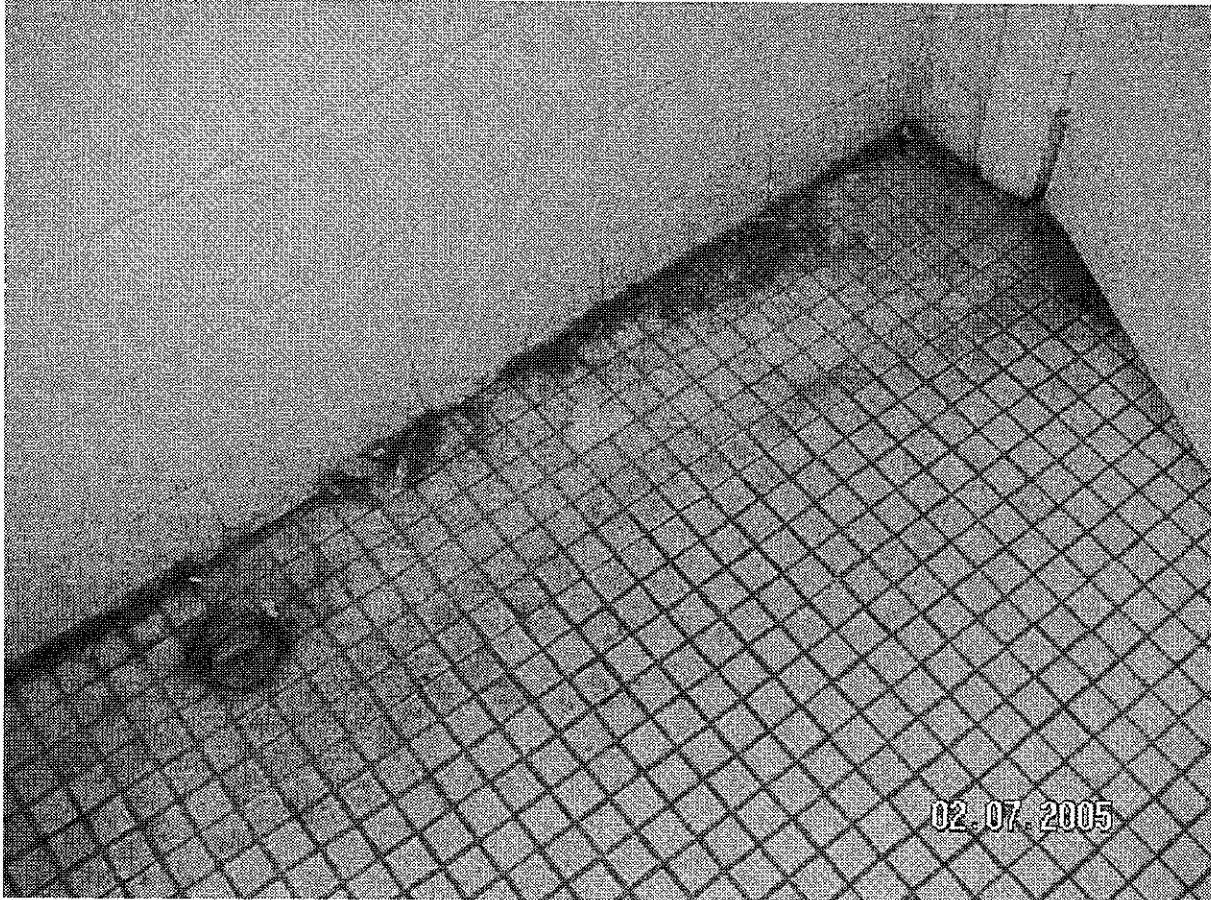
Fig. _____. Dust contamination in bathroom 904 (9 th floor). Janitor has not properly cleaned this bathroom for years. The whole building is contaminated with dust. To this day bathrooms, hallways and walls on 9 th floor are contaminated with large amounts of dust, which is a health hazard. This fact contributes to tenants getting lung infections. Two tenants on 9 th floor were treated twice this year 2007, for respiratory infections. Capitol Hall S.R.O. Dated: February 7, 2005.
