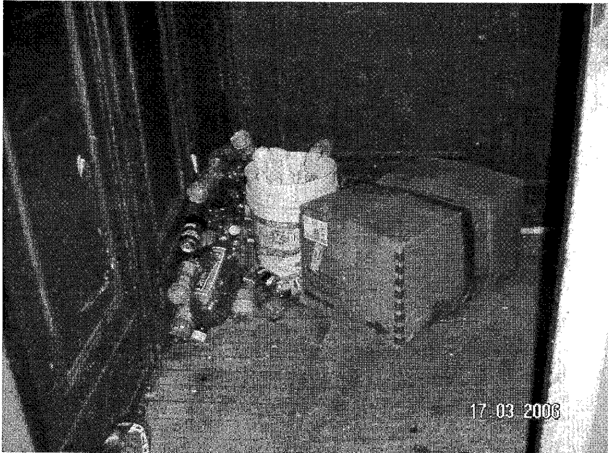
Fig.____. There are only two elevators for 203 tenants. But only one elevator is used as a passenger elevator. Many times the passenger elevator breaks down and the tenants are forced to use the service elevator in this condition (above). Service elevator full of empty cans and bottles in Capitol Hall S.R.O. – to this day, 2007. Dated: March 17, 2006.
