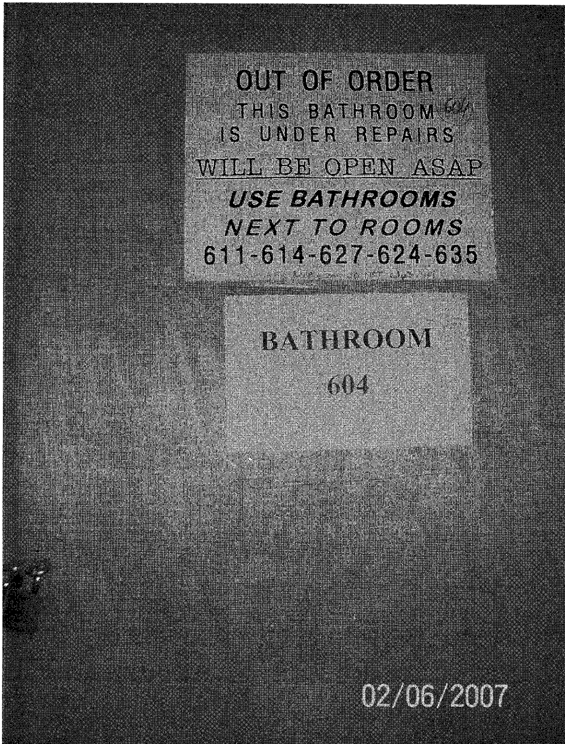
Fig. ____ . Common use bathroom 604 (6 th fl) is padlocked and kept inaccessible for the tenants. Landlord refuses to repair the common bathrooms and has a policy of not fixing them for months or even years. Director of the residence, Mr. Howard Fleishman and Adult Protective Services lie blaming tenants for “flooding the bathrooms”. Capitol Hall S.R.O. Dated: February 6, 2007.
