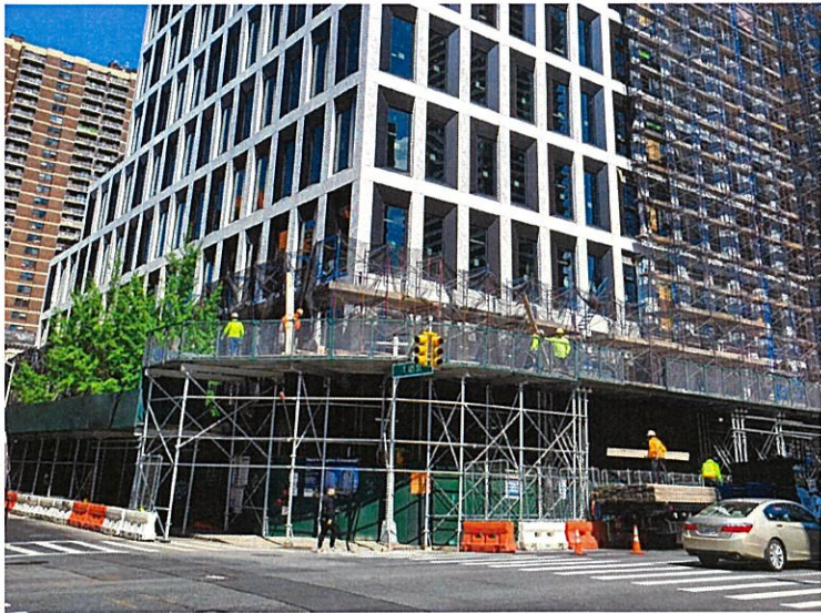
1. View of the Development Site facing northwest from the intersection of Third Avenue and East 121st Street.
