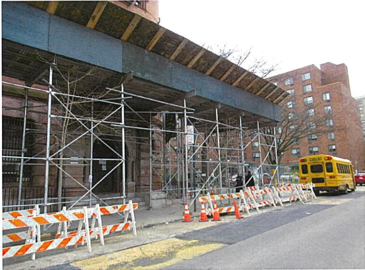
10. View of the south side of East 121st Street facing southwest from the Development Site.
