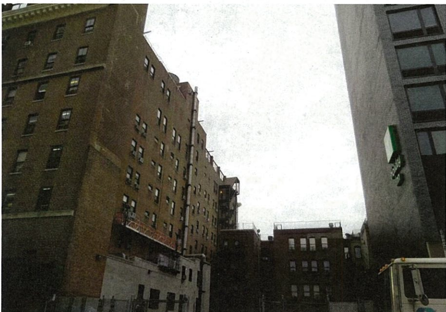
1. View South of West side of building from Schermerhorn St. Photograph taken on: 02/10/2016
