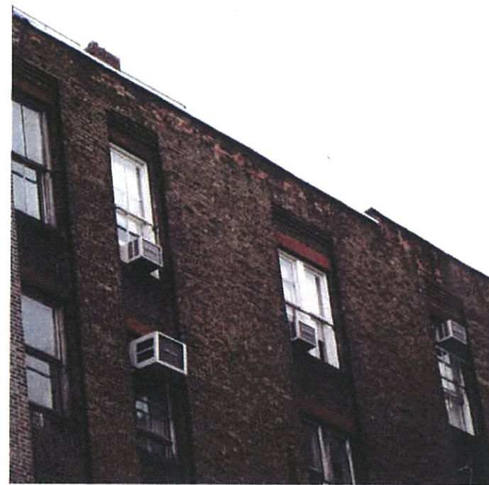
6 SOUTH ELEVATION, SOILING & DETERIORATED MASONRY PHOTOGRAPHED: 01.20.15
