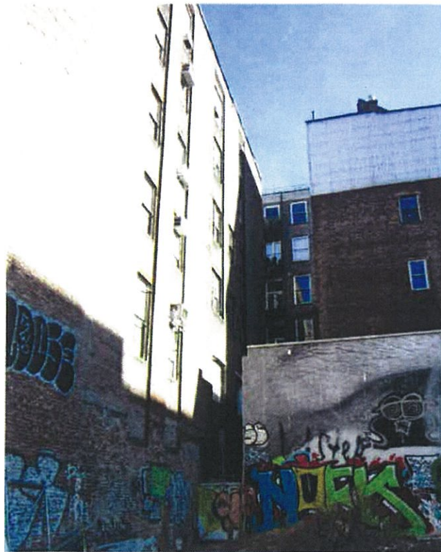
1 SOUTH ELEVATION, GRAFFITI & OPEN JOINTS PHOTOGRAPHED: 01.20.15
