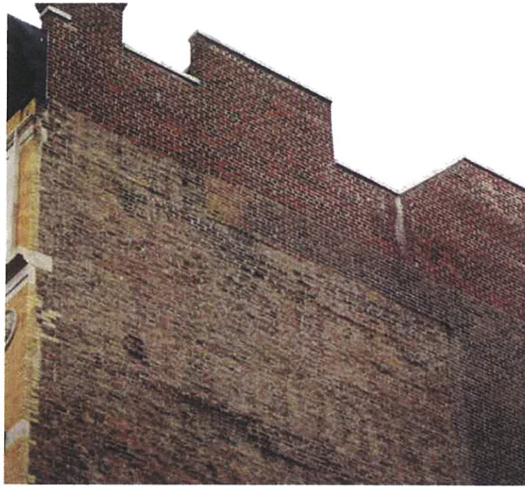
5 SW CORNER OF BUILDING, OPEN JOINTS & PREVIOUS REPAIRS PHOTOGRAPHED: 01.20.15
