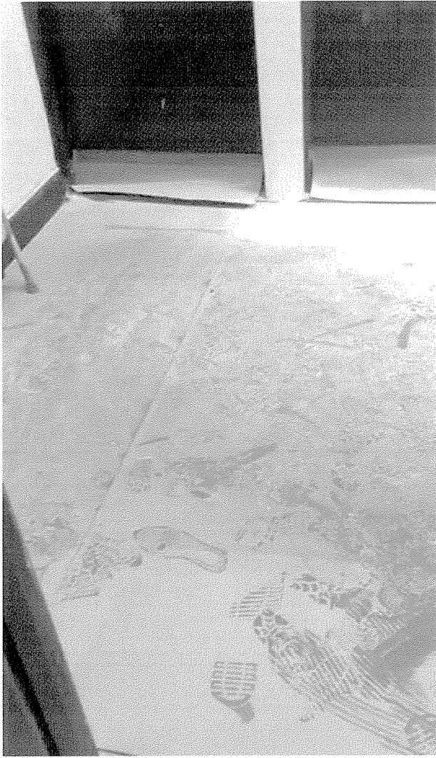
Construction Dust in hallways
