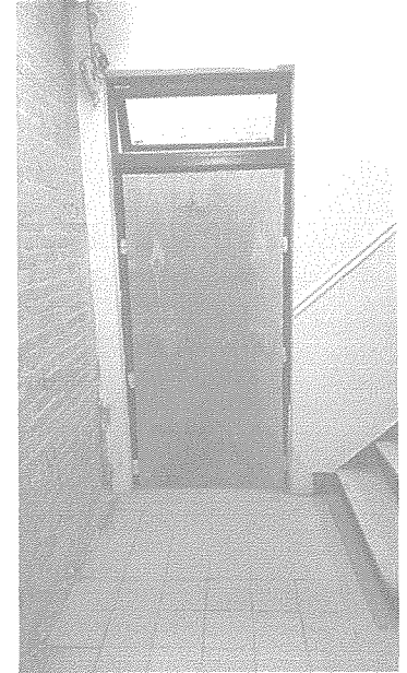
Fire door permanently shut
