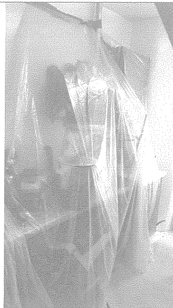
Construction in occupied tenants apartment to accommodate new apartment upstairs with luxury appliances (washer, dish washer), tenant told that he couldn't use kitchen for several days, 1 days notice
