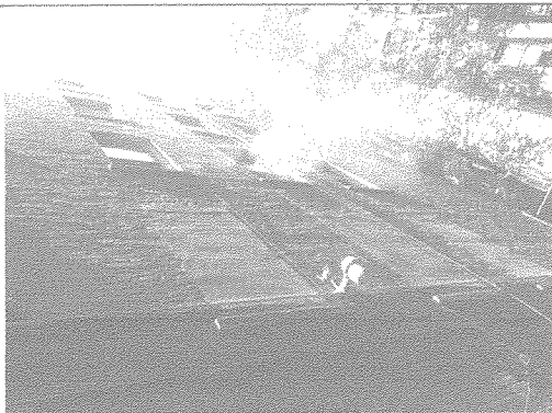
Construction dust pouring out of windows
