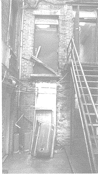
Back of fire door permanently blocked, with just a piece of wood, tied up
