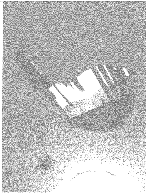
Hole put in tenants apartment ceiling, accidentally, worker was injured (head injury) and was told not to seek medical attention by boss on construction site
