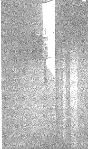
Fire door on roof that doesn't work, open at all times of the day/night
