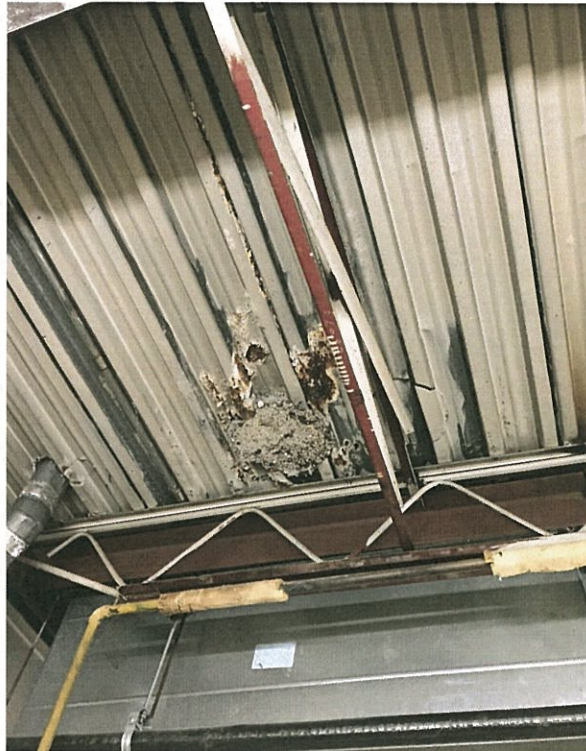
Water damage at Clinton Hill Library, Brooklyn
