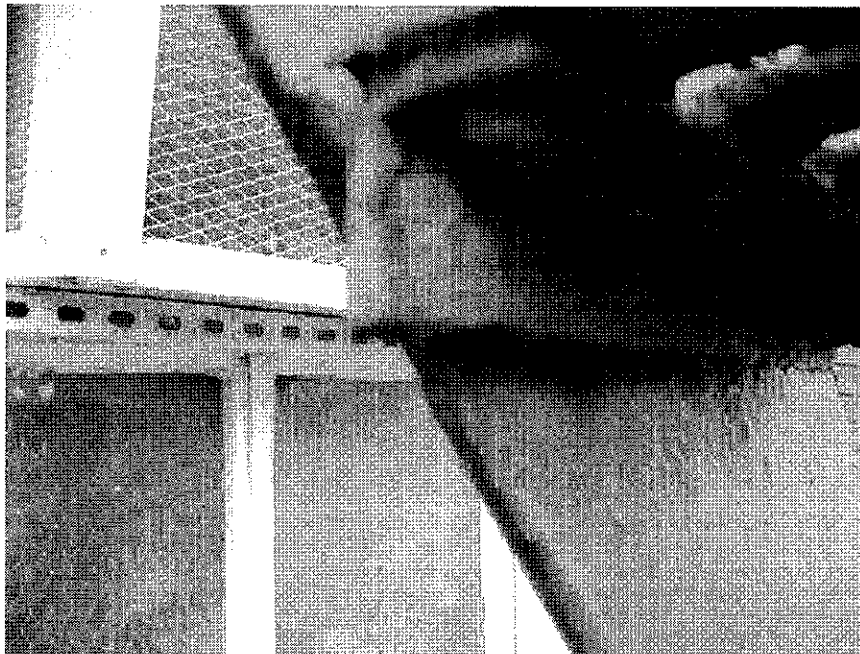
Photo 6: Missing Bolts at the Fire Escape Stair Step Support
