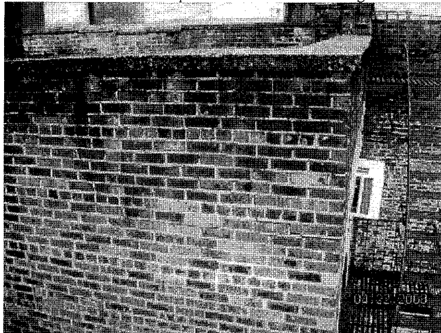
Photo 9: Stepped Crack at the rear corner
