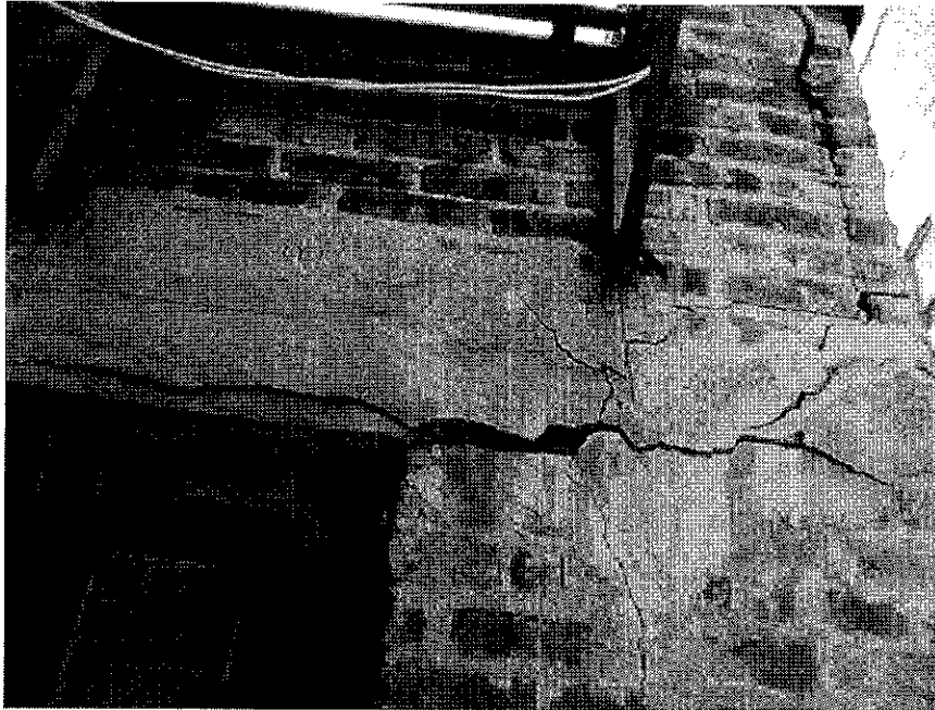
Photo 3: Corroded Steel Lintel and Cracked Masonry Wall
