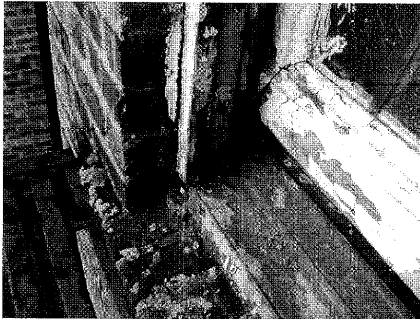
Photo 1: Typical Wood Window in Poor Condition
