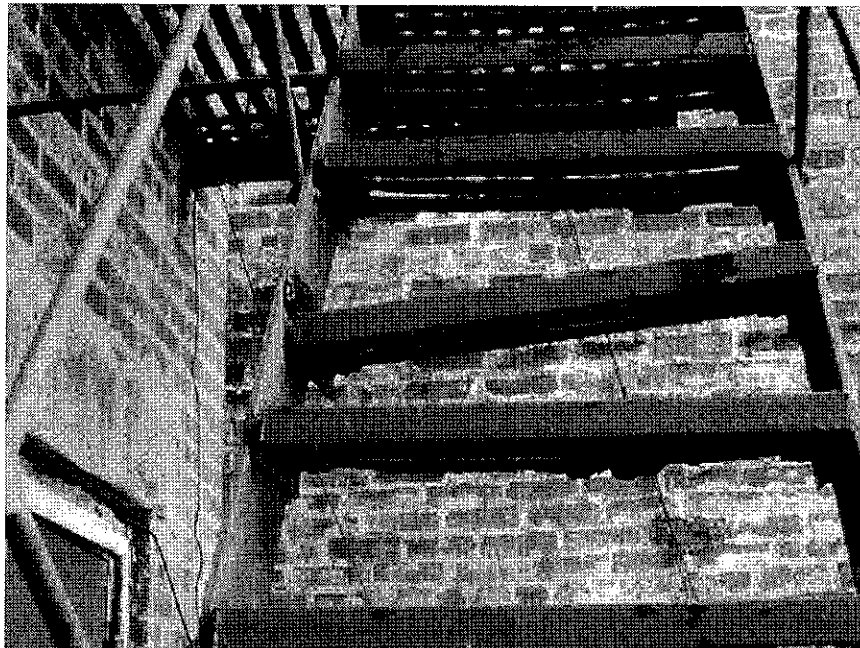
Photo 4: Deteriorated Steel Fire Escape Steel
