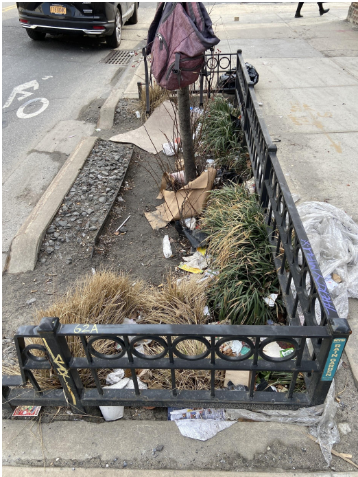
A denuded, trash-filled rain garden in Newtown Creek watershed. Inlets are clogged with sediment, which impacts the ability of the feature to absorb and treat stormwater.
