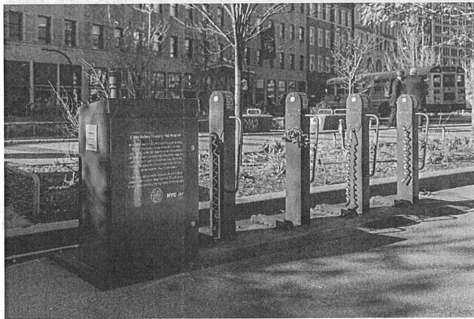
Public E-bike Charging Stations at Cooper Square, Manhattan
