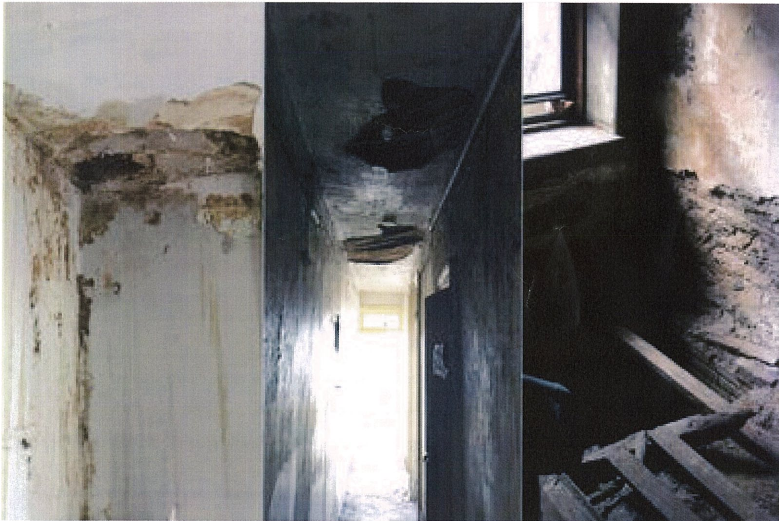
In vacant apartments residents say mold is "rampant" and that the basement is in disrepair.
