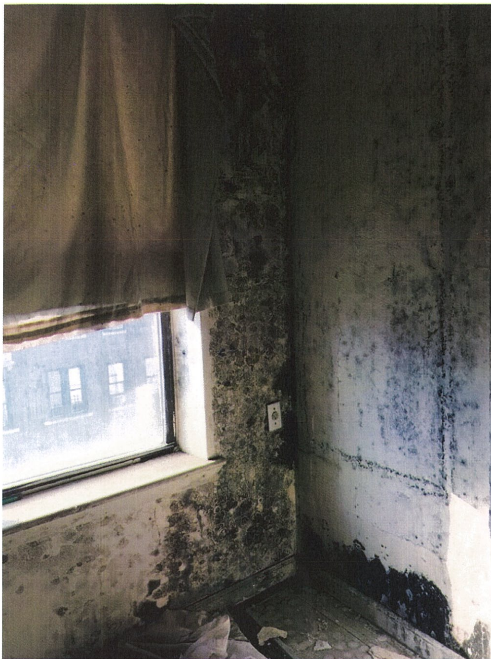
Mold covers the wall of a vacant apartment. (Joseph Jaafari/Gothamist)
